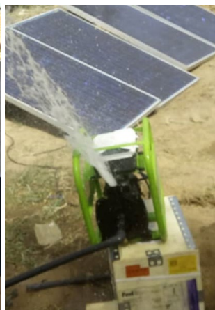
Pump connected to panels
