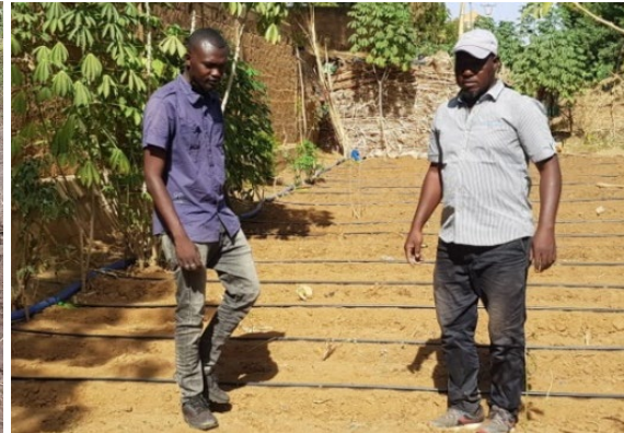
The HGT team during the installation of the drip irrigation system at lead farmer Mariama Tinni.
